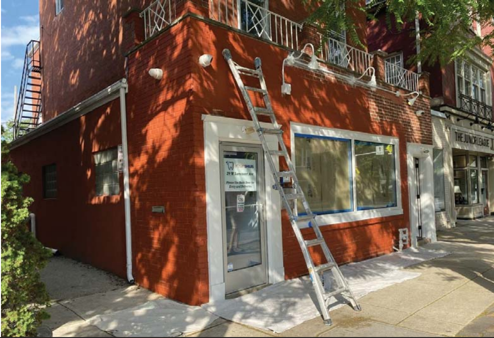
Work was stopped when the unapproved painting work was observed
